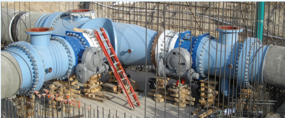
Two 48" EKN® Butterfly Valves — shown here being installed on the North Shore Aqueduct in Utah — help to safely modulate and control gravity flow in the aqueduct system.
